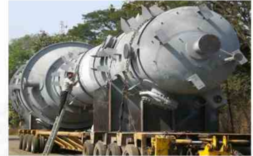
Column Internals & Revamp
