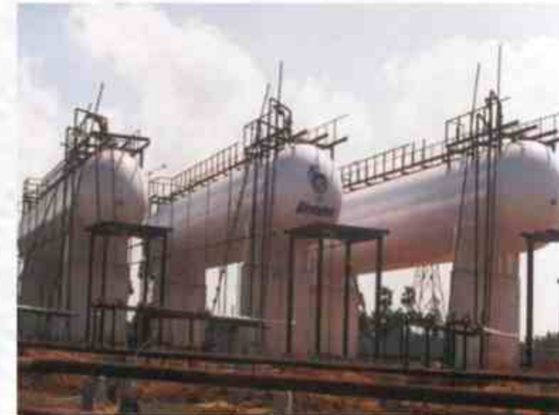
Bullets – Mounded Storage & Above Ground Bullets
